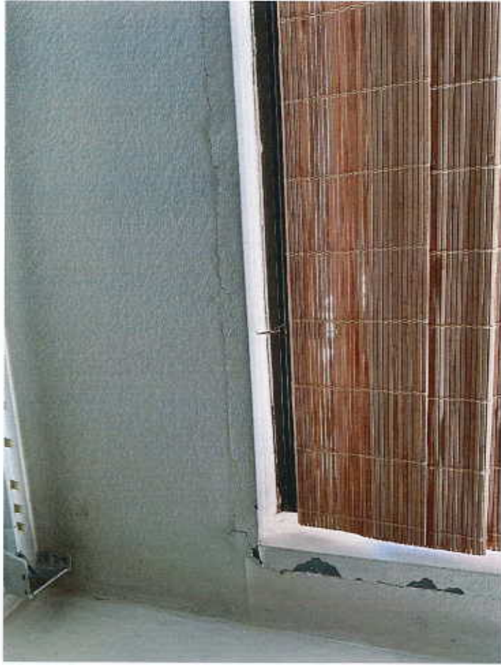
CRACKS IN DRYWALL ABOVE WINDOW AND ALONG THE LEFT SIDE
